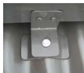
Close up of a mounting bracket fixed to a corrugated iron roof.
